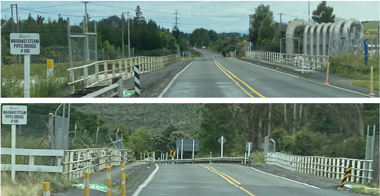
An example of missing bridge end markers on both ends of Wairakei Steam Pipes Bridge on Wairakei Dr.
