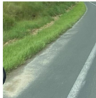
Example of high shoulder that caused water to pond
