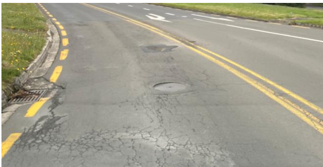
Example of extensively cracked AC
