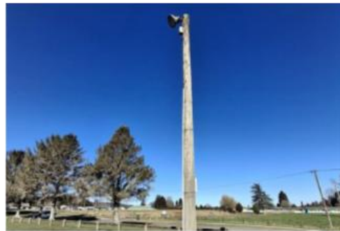
Not working: Existing timber light pole and single fitting near the roadside boundary.
