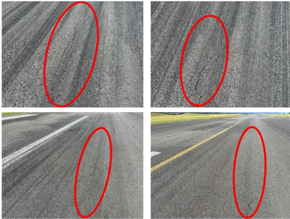
Figure 3-2: Main Runway – Crocodile cracking
