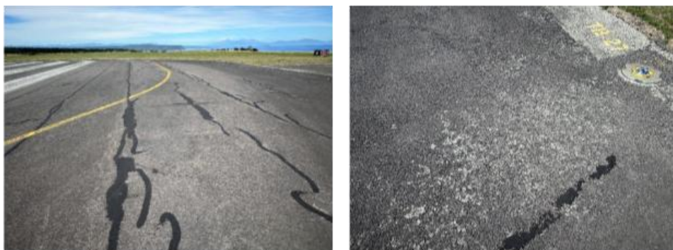
Figure 3-6: Main Runway – Accelerated weathering, white staining, aggregate loss
