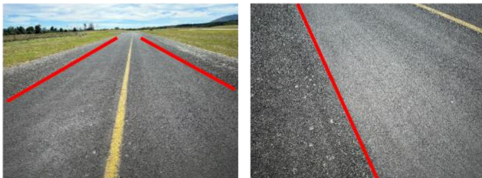
Figure 3-9: Taxiway A (widening) – Debonding, lichen growth
