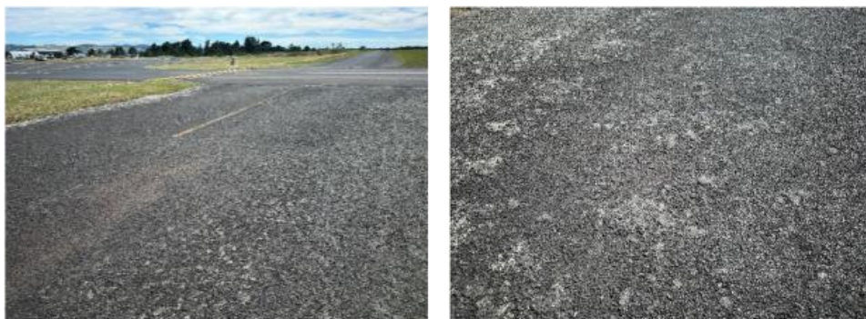
Figure 3-11: Taxiway C – Loose aggregate, red algae, Lichen
