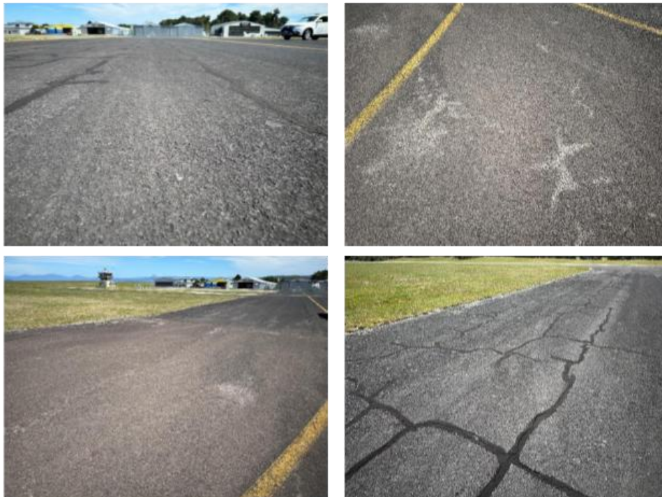
Figure 3-12: Taxiway D – Cracking, ageing, weathering
